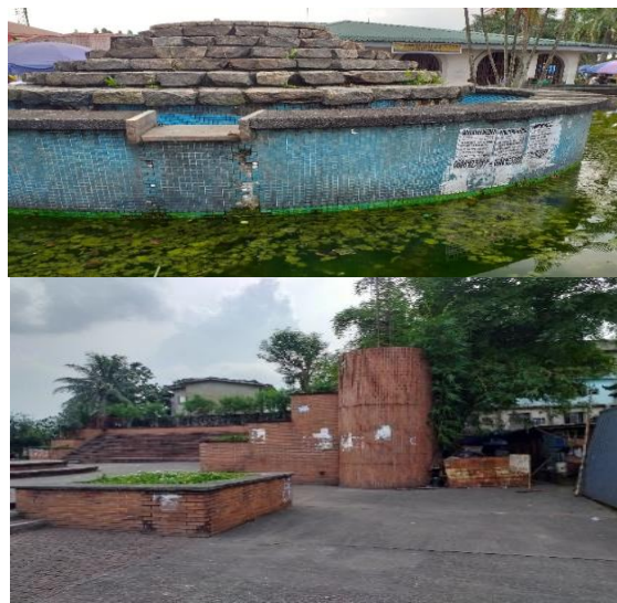
Plate 1: Infrastructural decay at Ibom Plaza Source: Author’s Fieldwork, August 2019.
