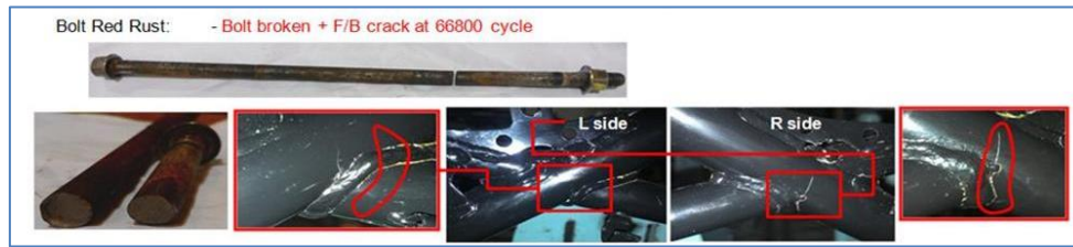
Fig-14: The results of the 10x250 bolt flange fracture and the frame body after the durability test
