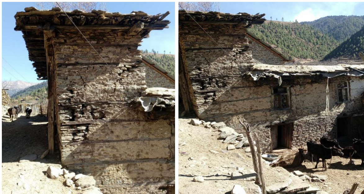
Picture 1: The common and repeated construction defects cracking on wall is seen. The wall may collapse due to uneven settlement from the foundation
