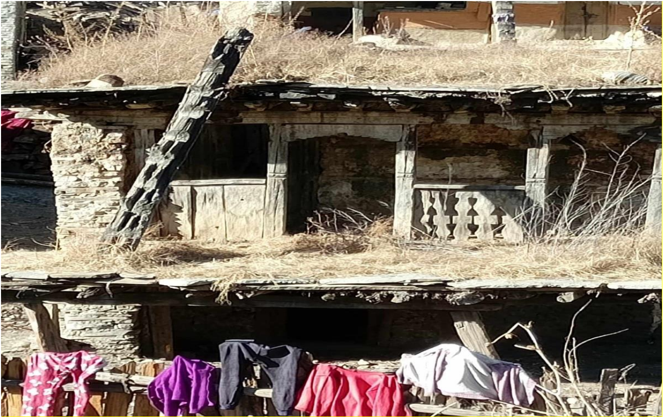
Picture 2: Due to settlement issues the level of window, door fall down from their original level
